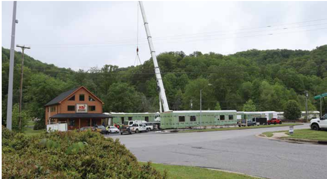
Cardinal Homes, a business of Kituwah, LLC., sets modules for their new office space on the morning of Tuesday, April 28. (BROOKLYN BROWN/One Feather photo)
