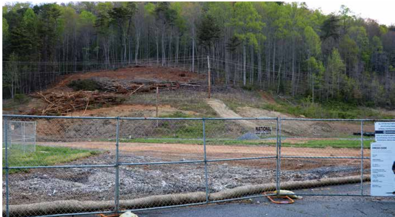
The Tribal Bingo Project is back on following a halt in construction that lasted a few weeks due to a right-of-way and easement dispute. The project site is shown in this photo taken Monday, April 13. (SCOTT MCKIE B.P./One Feather photo)
