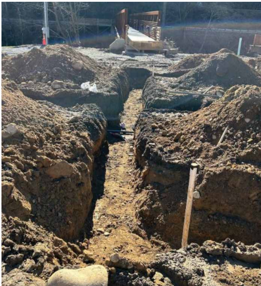
Construction is ongoing for the new water features in the Horseshoe Area of downtown Cherokee, N.C.
