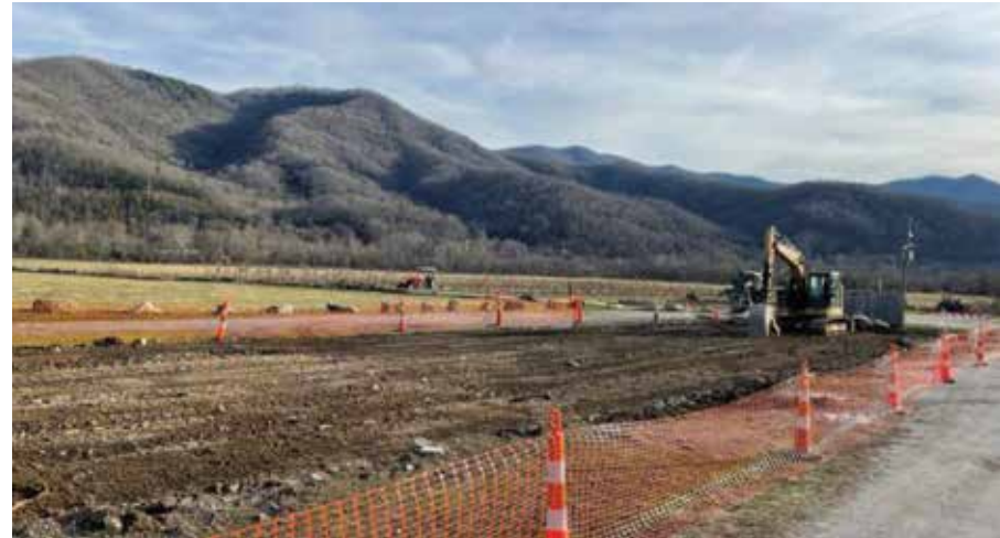
Construction work has started on the new Kituwah Hangar Project. (Photos courtesy of EBCI Project Management)
