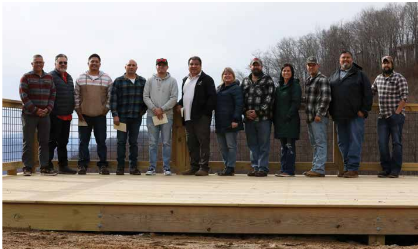
Tribal officials of the Eastern Band of Cherokee Indians (EBCI) held a groundbreaking for improvements to the Soco Falls Trailhead on the afternoon of Friday, Dec. 13. Shown, left to right, are Ugwyiyuhi (Principal Chief) Michell Hicks, Dinilawigi (Tribal Council) Chairman Mike Parker, RJ Arneach, Wayohi (Wolftown) Rep. Bo Crowe, Aniwodihhi (Paint-town) Rep. Michael Stamper, Elawodi (Yellowhill) Rep. David Wolfe, Becky Bowe, Yancey Jones, Kim Deas, Zack Hicks, Justin French, and Brett Smith. (SCOTT MCKIE B.P./One Feather photo)
