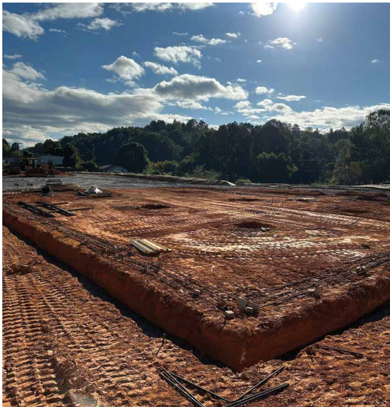
After a brief delay, construction officially commenced in September on the new Cherokee County Clinic site, a satellite clinic of the Cherokee Indian Hospital Authority (CIHA) that will serve enrolled members of the Eastern Band of the Cherokee Indians (EBCI) in Cherokee County. (Photo courtesy of Cherokee Indian Hospital Authority)
