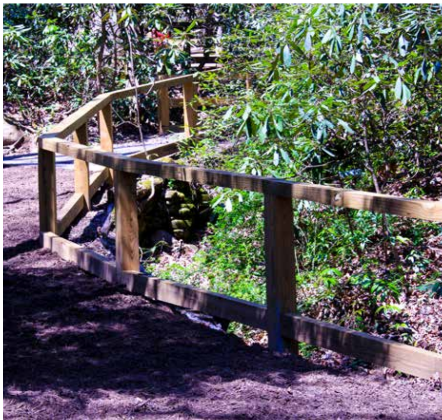
RAILING ABOUT IT: New, treated wood railings replace old, rotten locust railings throughout the Village. Some of the railings have been removed in places to further open up the area.
