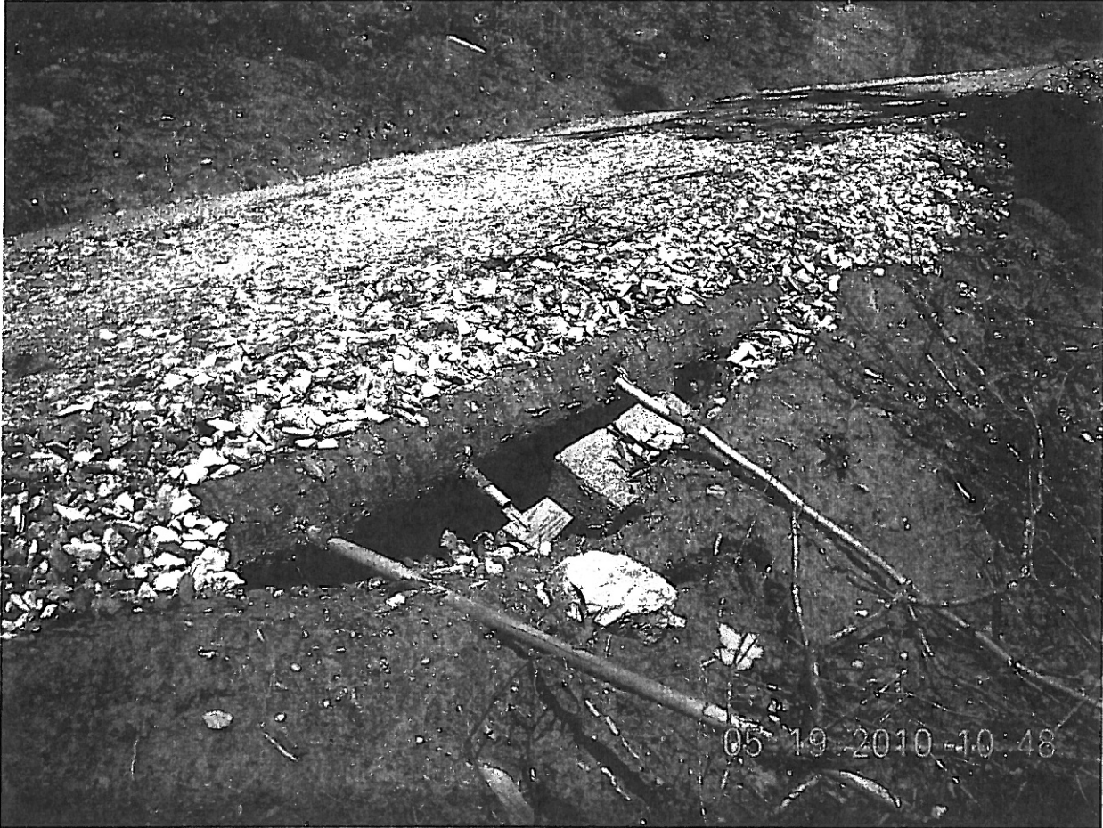
Homeowners attempt to stop erosion.
