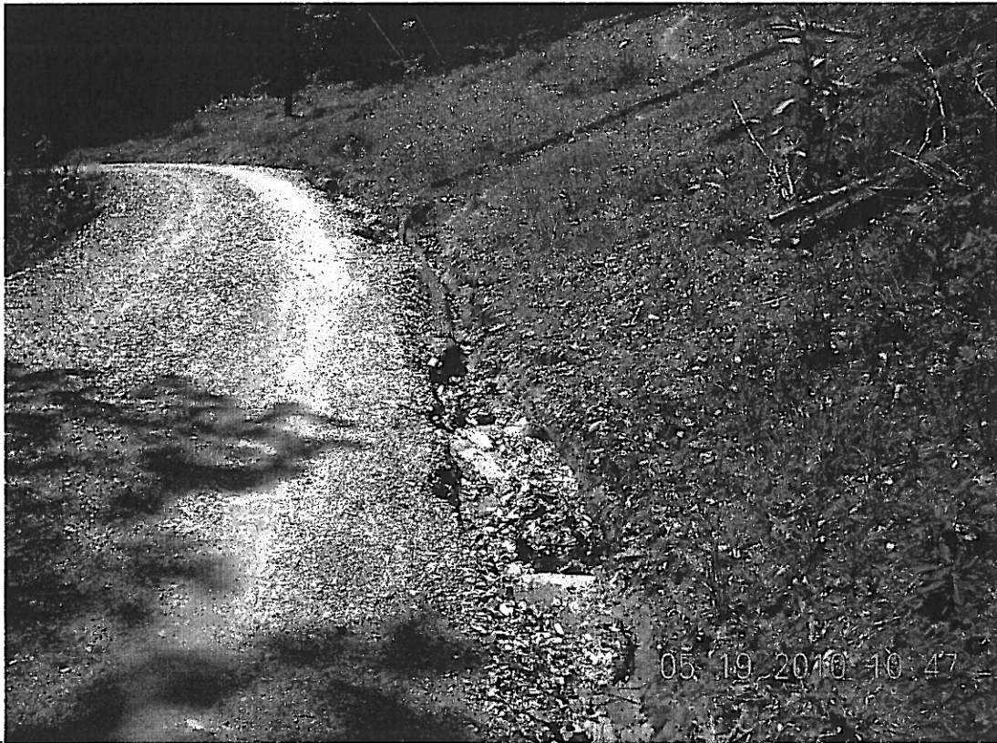
Pictures showing erosion of ditches at top of
